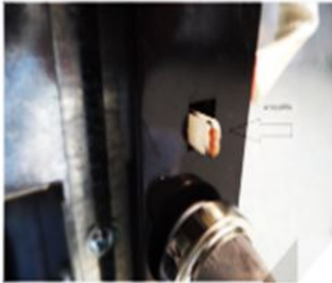
Smoke sensor is accessible
